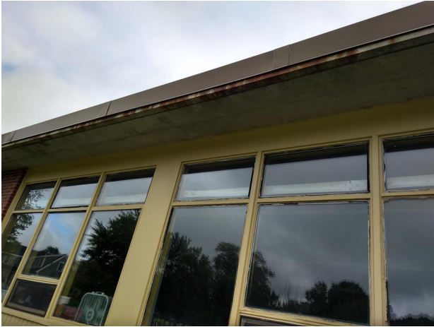
7. Original roof soffits have corroded.
