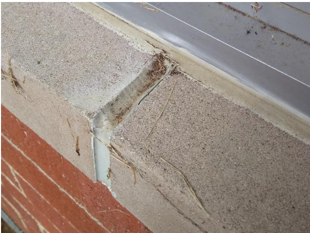
4. Some sealant shows early signs of deterioration.
