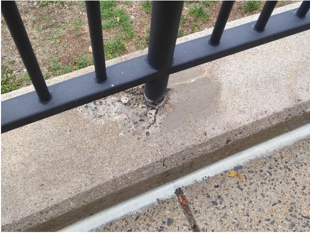
1. Concrete has spalled at some rail posts.
