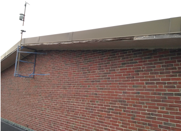
13. The fascia is rotted at the Cafetorium.
