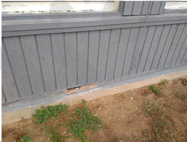
5. The wood siding is rotted and damaged.
