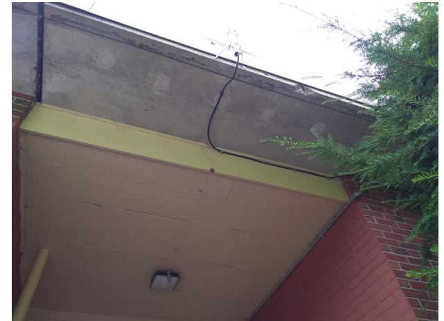
6. The concrete facias and soffits have spalled.
