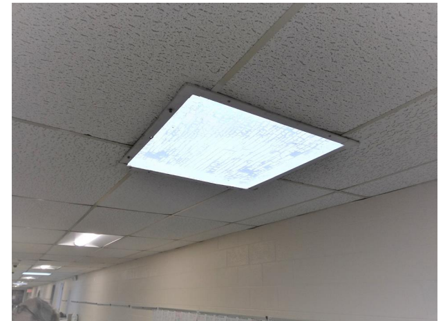
18. The skylights in the corridors are damaged.
