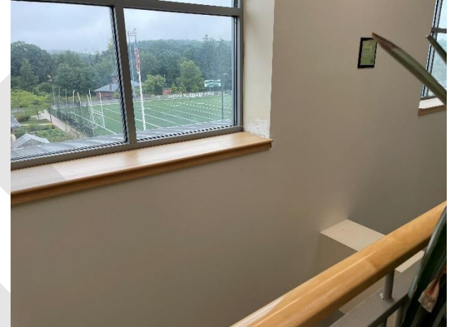
9. Several windows show signs of water damage.
