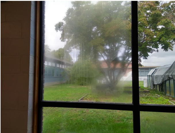
4. Thermal pane window has seal failure.
