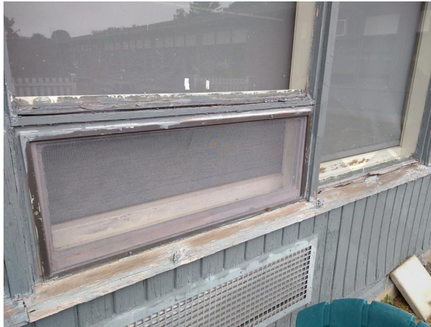
2. Original windows and trim have deteriorated.
