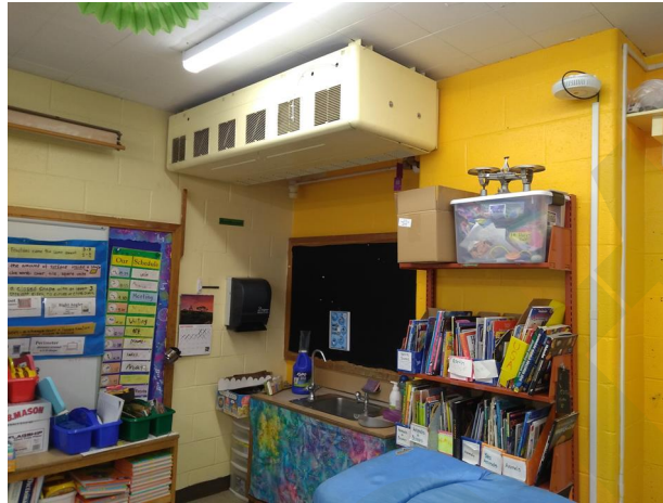
20. Classrooms have outdated and inefficient unit ventilators.
