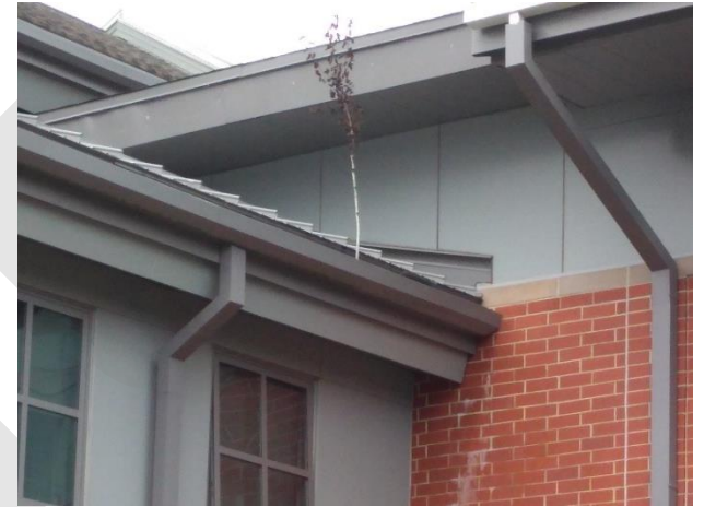
3. Some gutters are clogged with vegetation.
